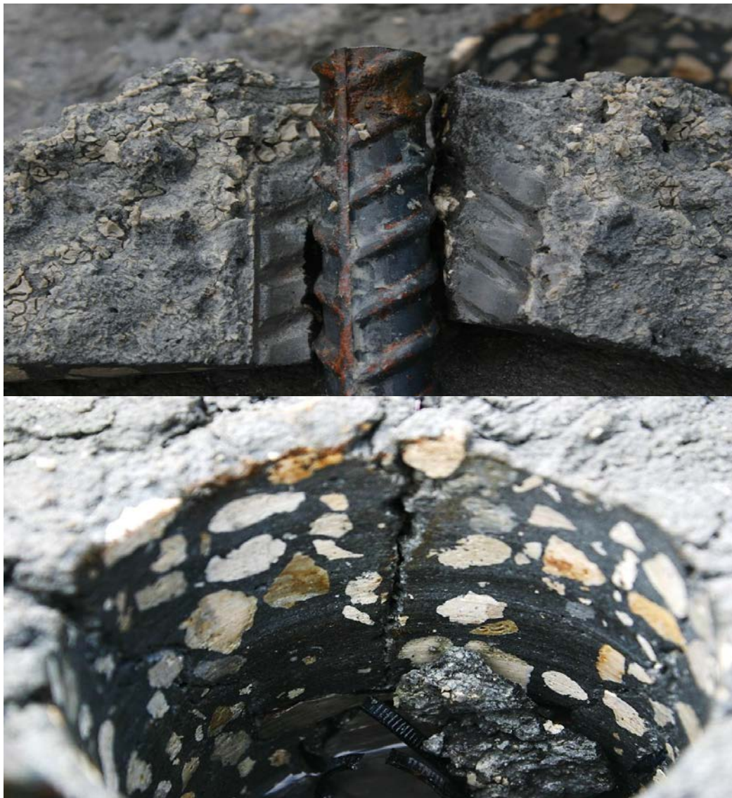
Figure 4.11. Slurry present at surface of reinforcement (top) depth of visible crease (bottom).
