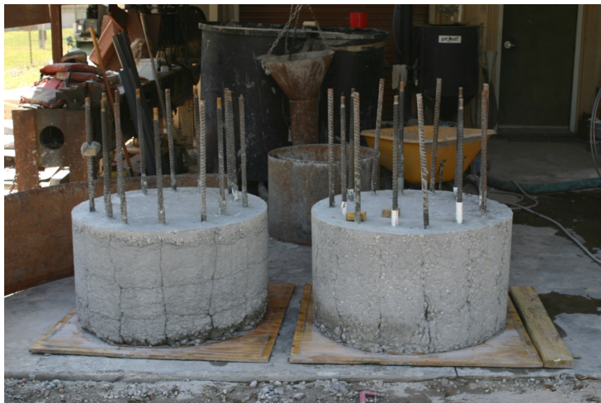
Figure A.13. Shaft 1 (right) and shaft 2 (left) after pressure washing.
