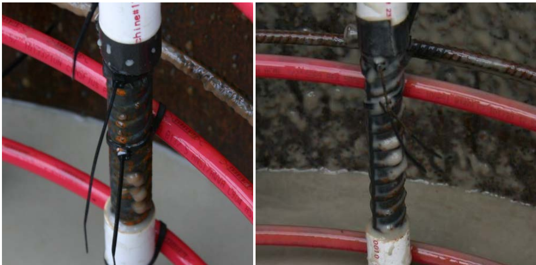
Figure 5.1. Residual slurry noticed on reinforcement 30 second (left), 40 second (right).
