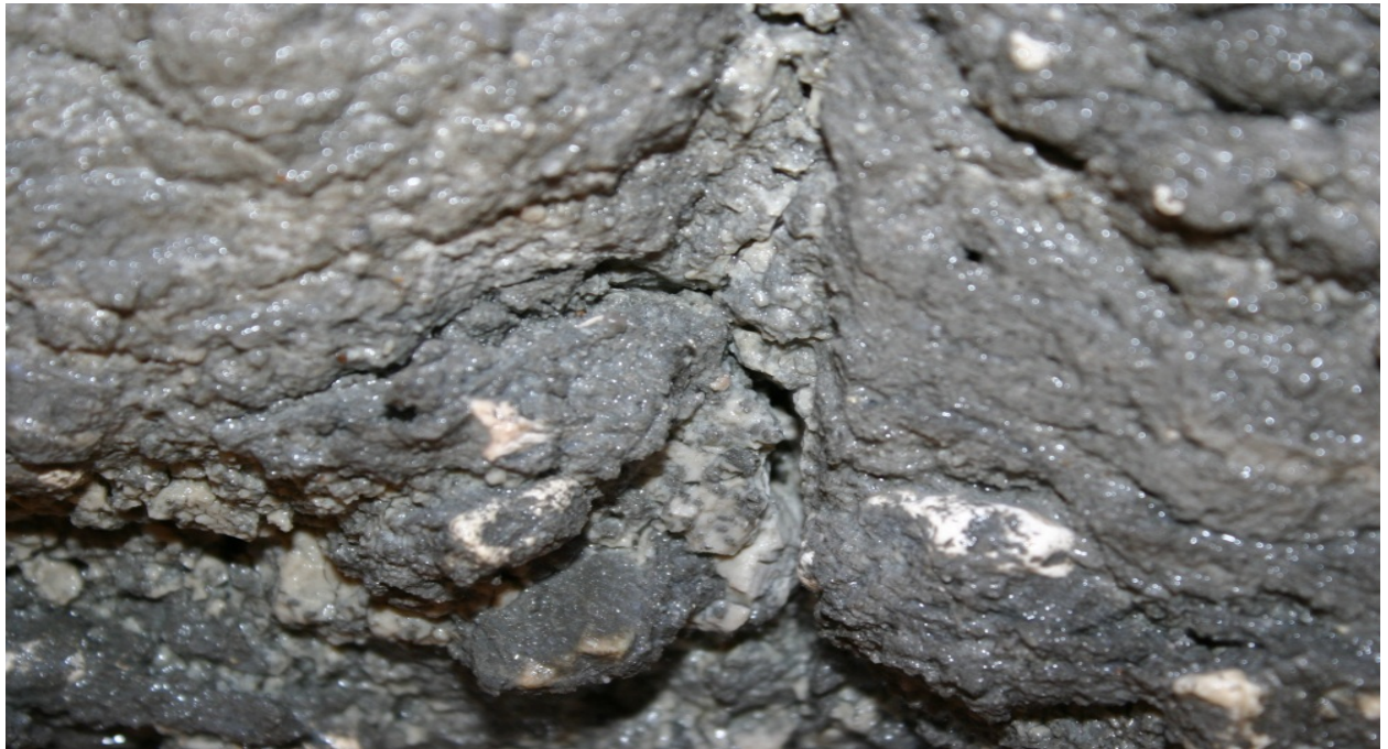
Figure 5.12. Slurry encased in void in 90 sec/qt shaft.
