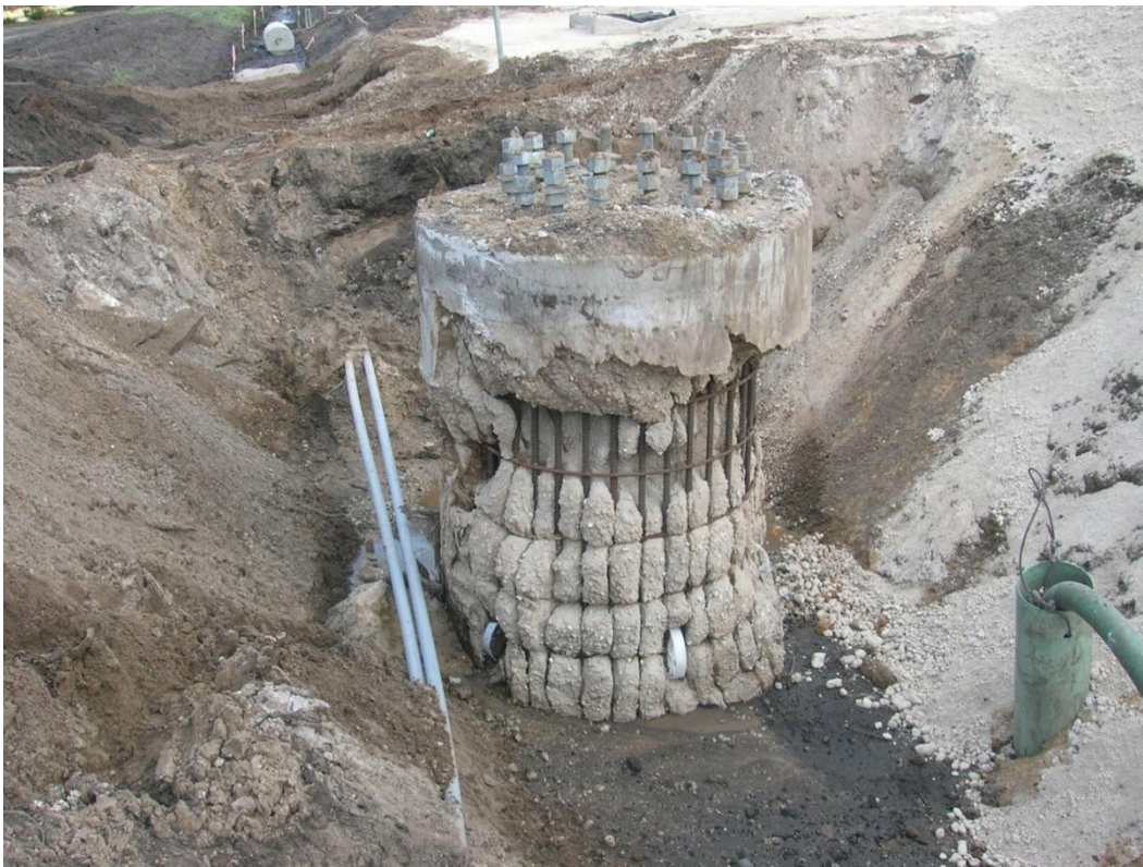
Figure 1.2. Shaft exhumed to show poor concrete flow performance from slurry or fresh concrete properties.
