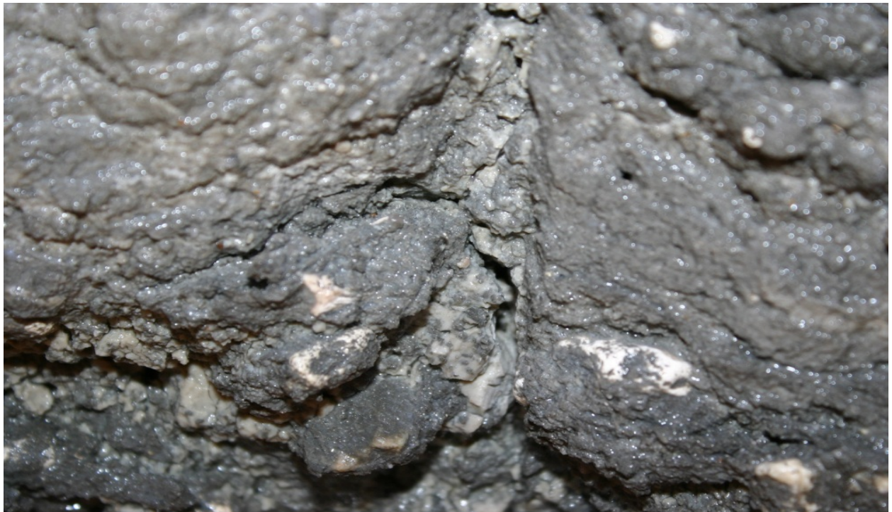
Figure 4.10. Slurry that was encapsulated in the concrete (90-second shaft).
