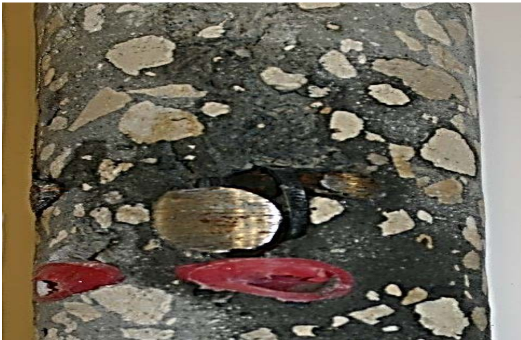
Figure 5.10. Poor consolidation around reinforcement in 40 sec/qt shaft.
