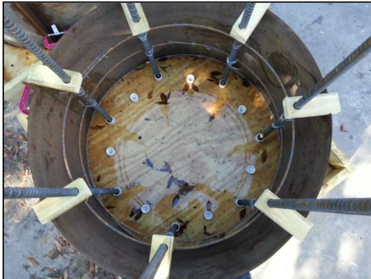
Figure A.5. Form with structural reinforcement prior to placement of pullout steel.
