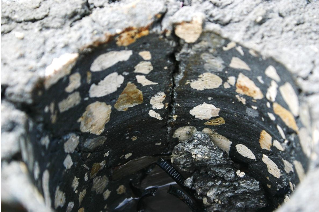
Figure 5.9. Core hole in 50 sec/qt shaft; crack corresponds to line formed by reinforcement.
